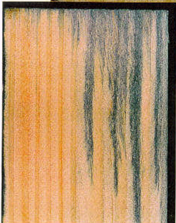
Moderately Deteriorated Fir 2 X
