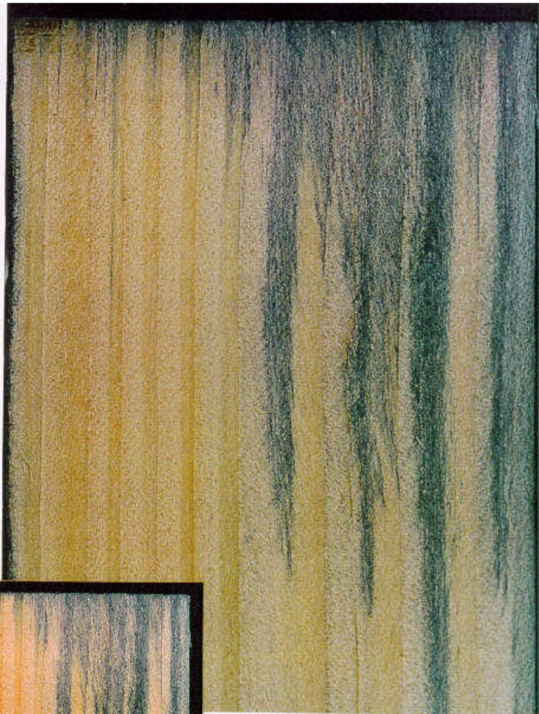
Moderately Deteriorated Fir 4 X
